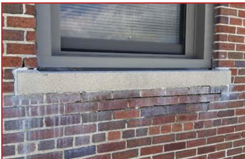
Masonry at the Elementary School in need of repointing.
