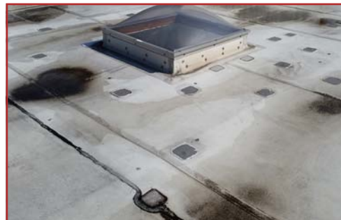
Roofs at the Junior/Senior High School in need of replacement.
