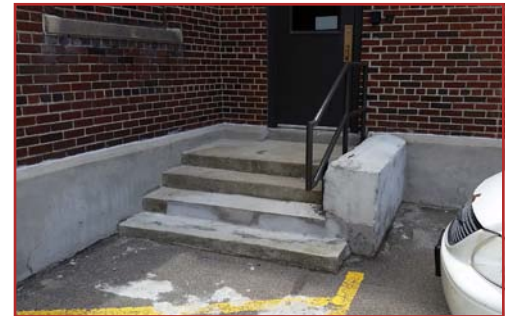
Stairs and entrances doors at the Elementary School in need of repair.
