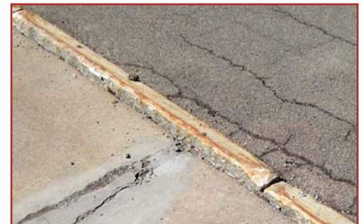
Sidewalks, curbs, and pavement at the Junior/Senior High School in need of replacement.
